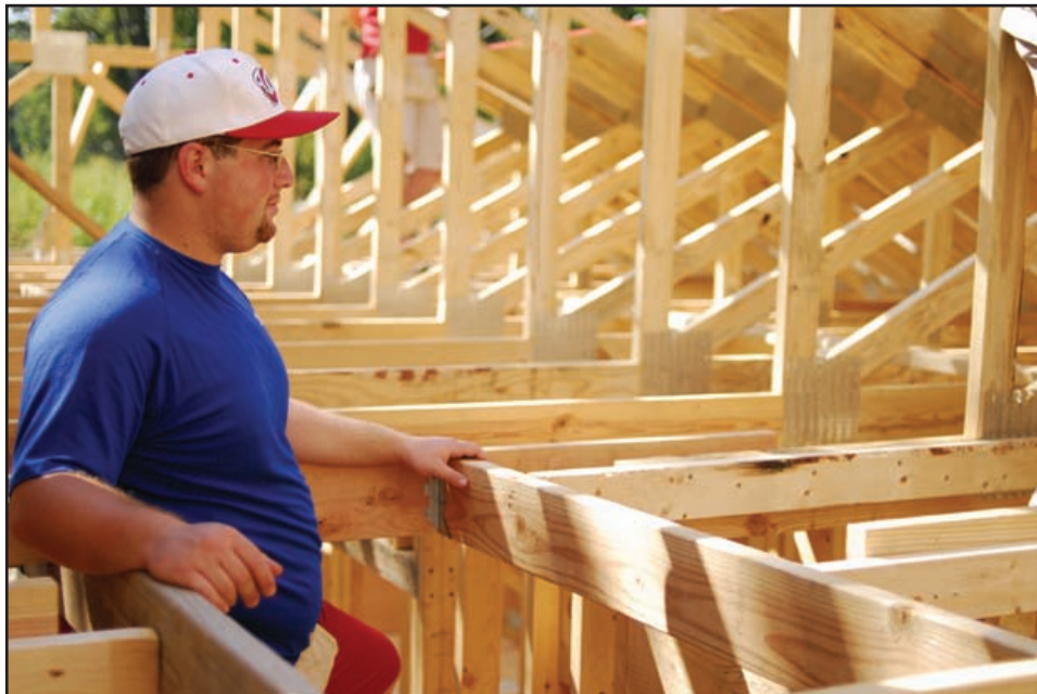
Top: Members of the Epsilon pledge class Ryan DeMeuth and Will Garcia work together to nail a board to the roof of a Habitat for Humanity home. Bottom: Zack Ryle pauses to observe the progress being made on the roofing project.
